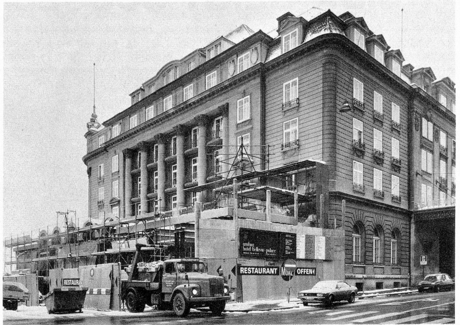
The new "city restaurant" under construction as part of the Sw.Fr. 5.5 million modernisation scheme at Berne's Bellevue Palace Hotel.
