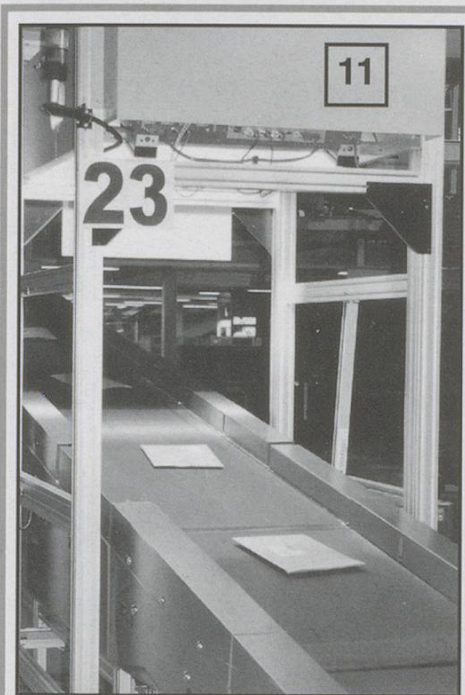
After the bar code has been read by one of these gates, the parcel will be conveyed with full automation. The centre can handle a maximum of 15,000 parcels an hour. These almost flat packets are parcels: the centre does not handle letters.
