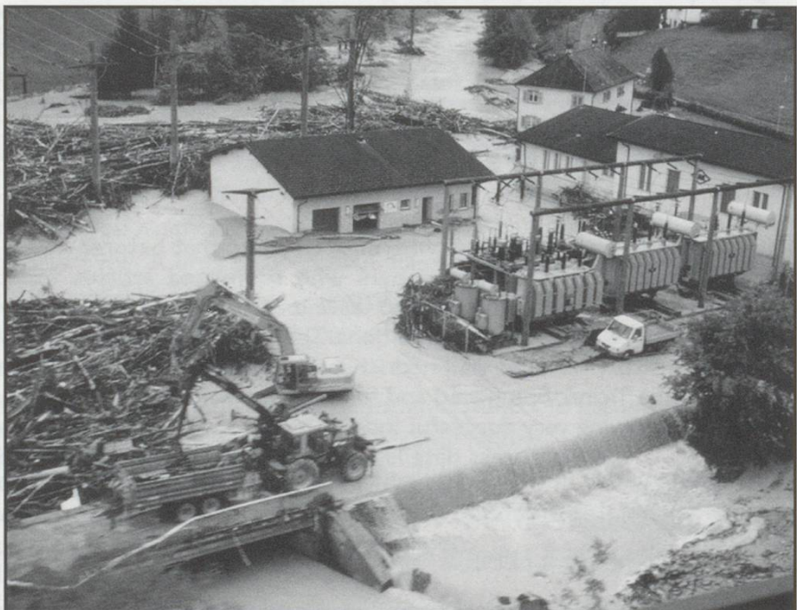
The electric power depot near Goldach, the morning after the flash flood. Taken from the train to St Gallen, 1/9/02 by Malcom Hardy-Randall
