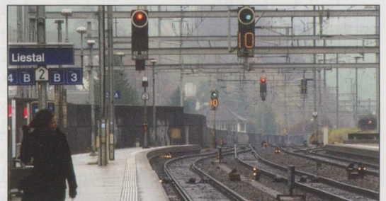
BELOW: Signals at Liestal. Platform 3 signal at stop, the through track clear to enter the section at 100 km. Note also the dwarf signals on the main lines.
