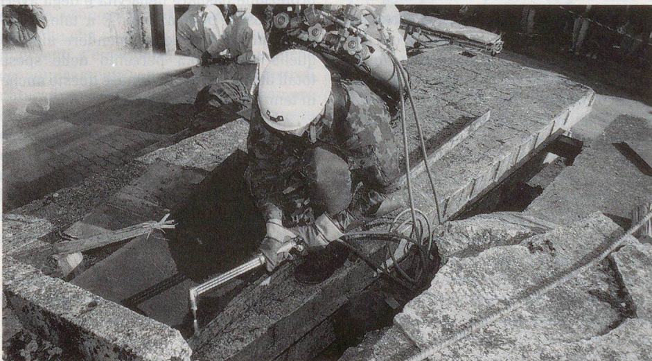
PHOTOS: RMINFO, PULLY
